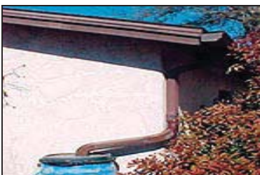
Catch rainwater from a roof w/ gutters
